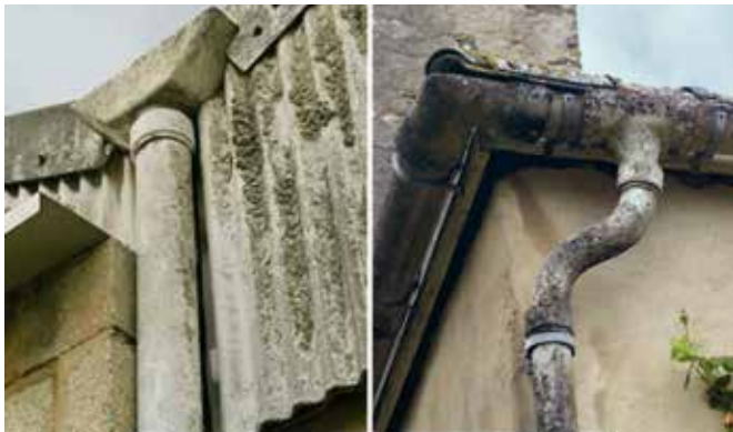
Asbestos cement downpipe and corrugated asbestos sheet
